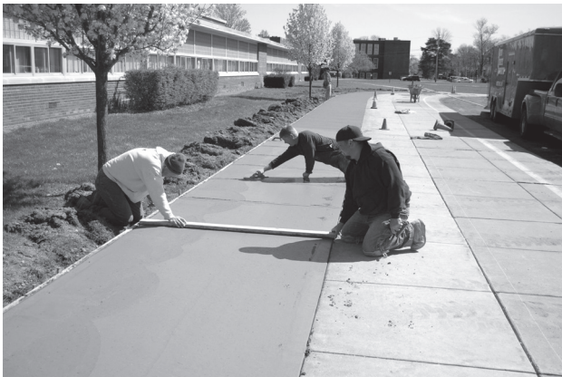
The local team from Martin Concrete Construction Company (based in Olmsted Falls) worked on the Falls-Lenox sidewalk expansion project over spring break in late March.
